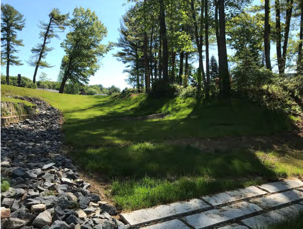
Fig 9: Slope above the manhole at Gundalow Landing/east side of the bay. Viewing east. (05-24-21)
