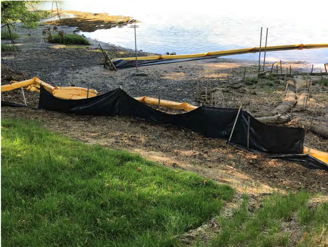
Fig 11: Toe of the slope at Gundalow Landing/east side of the bay. Viewing south. (05-24-21)
