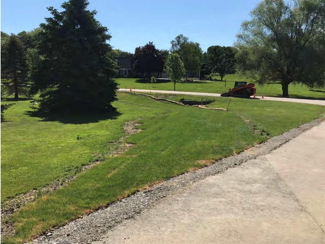
Fig 13: Sod applied over loam and flowable fill at 29 Gundalow Landing. Viewing east. (05-24-21)
